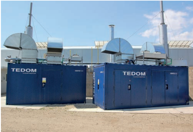
Biogas Plant Suchohrdly (CZ)
