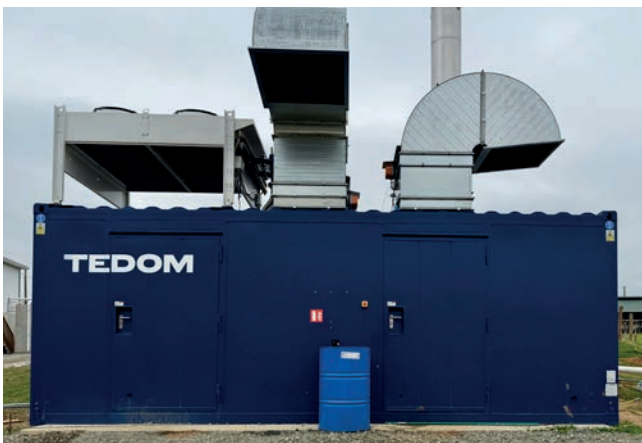
Biogas Plant Long Green Farms (MD)
